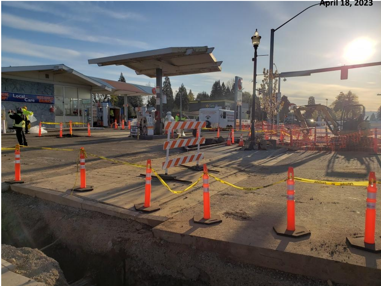
Cleanup on April 14, 2021, of a gasoline leak at the intersection of Main Street and Highway 99 in Monmouth. [Oregon Department of Environmental Quality]
